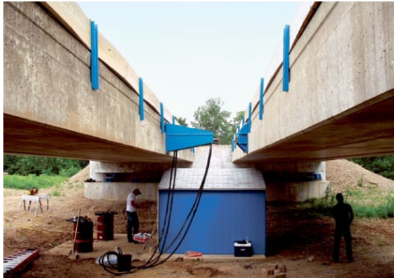
Quake Summit 2011 included a field trip to UB/MCEER's ECLIPSE campus to view a full-scale bridge test of elastomeric seismic isolation bearings that support these 72-foot long concrete box girder bridges
